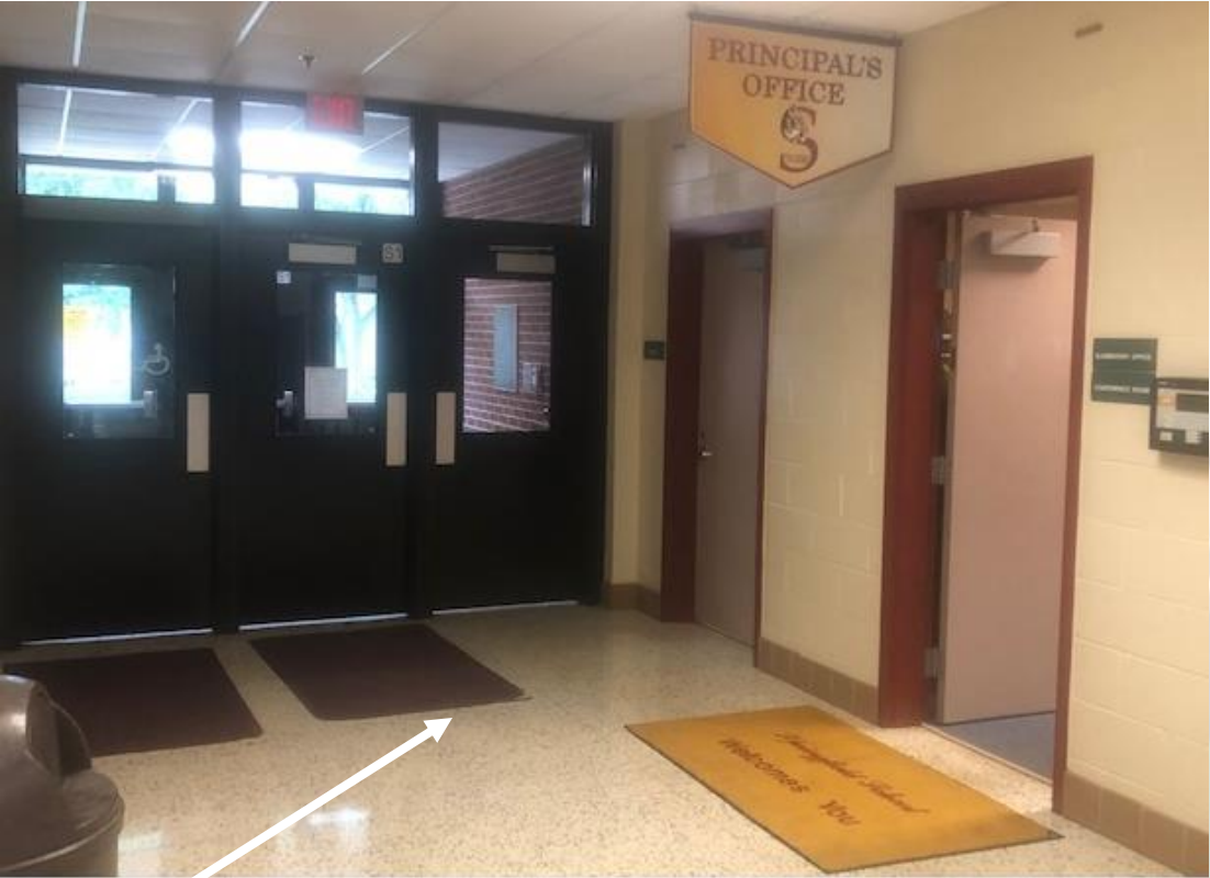
This is the entrance S1 by the elementary principal office. After visitors are “buzzed” in, they can access the elementary without. This construction design is from 1994 and is one of the most recent section of our school. At that time, school’s were not built with the safety features sought after in today’s school buildings.
